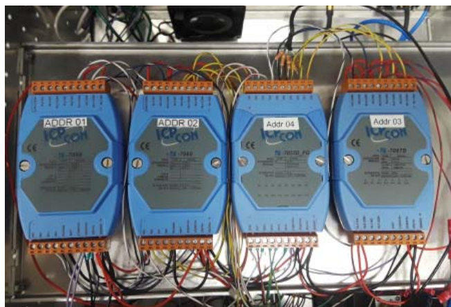
FIG. 2. Four digital input/output modules inside the RF Attenuation and Switching unit.
